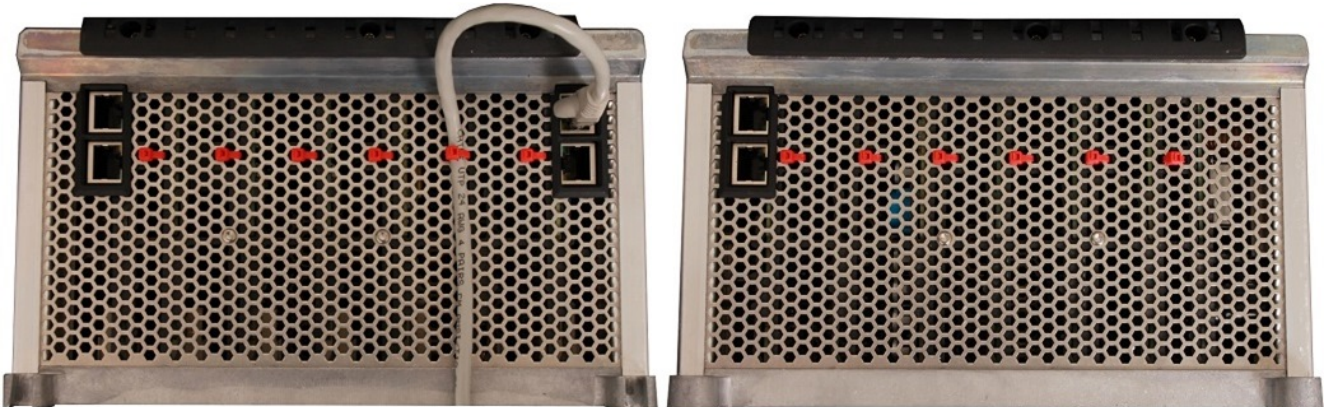
Figure 3.2 Cable tie slot positions shown by red cable ties (top of rack on the left; bottom of rack on the right, with an Ethernet cable example)
